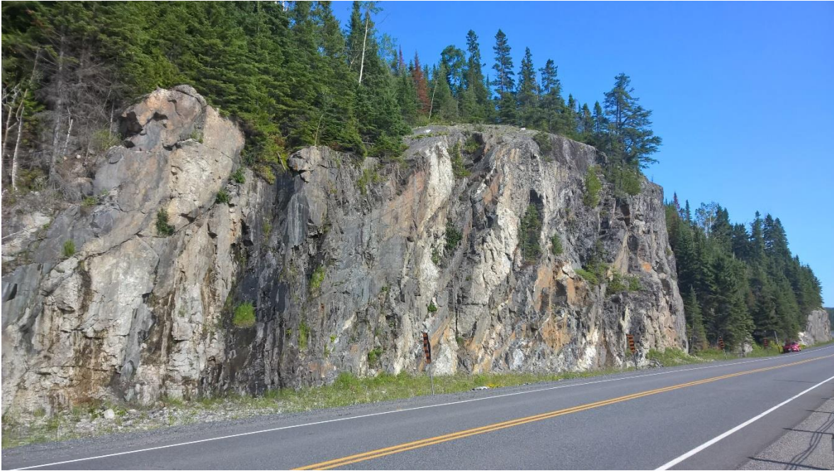
Figure 1 – Photo of the road embankment from similar rocks in the area; here a vertical slope with a height of over 15 metres.
