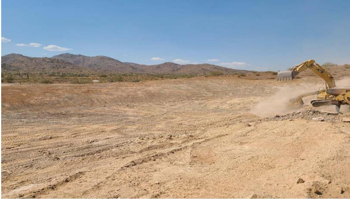
North Side of Leach Pond – Continuing Final Removal of Material and Rough Grading
